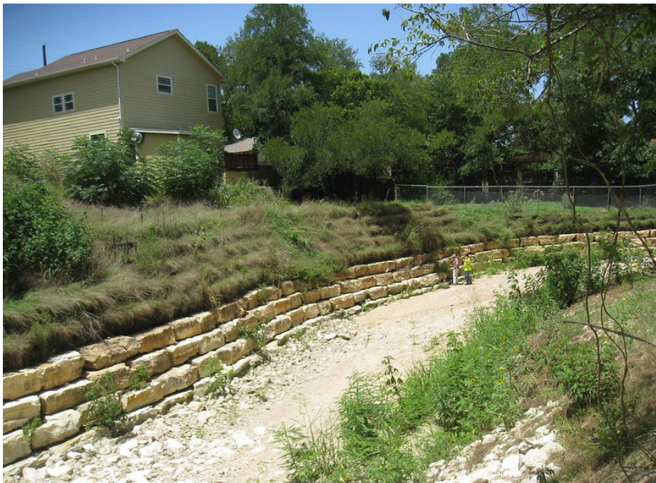
Streambank Stabilization in Austin, TX. Image by City of Austin Watershed Protection
